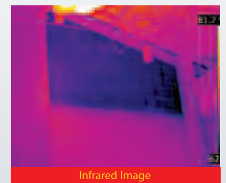
Fusion Image Showing Missing Insulation
